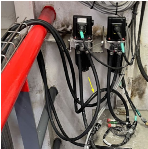
DEF hose with excessive length and loop
